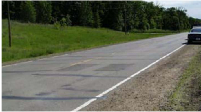
Figure 3: Transverse rumble strips (30)
